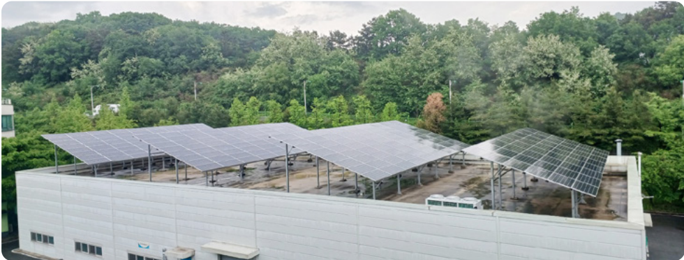
Choongju Plant Solar Power Facility
